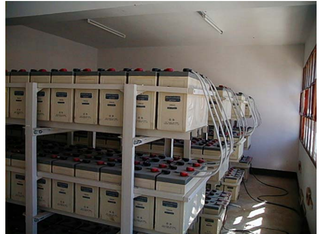
Fig. 16. GFMU 2 V 600 Ah VRLA in battery room.
